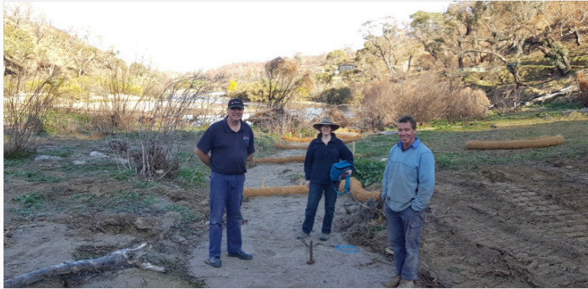
NSW Soil Conservation Service Operations Manager for Monaro, Ashley Bolton on site with landholders Lyn and Justin installing coir logs to prevent sediment flowing into the Murrumbidgee (photo courtesy of Antia Brademann)
